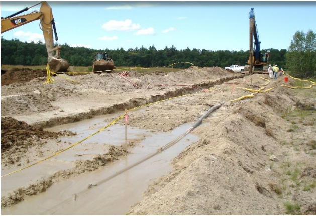
Above: Installation of the barrier wall in between Plow Shop Pond and Shepley's Hill Landfill. The barrier is about 40 feet deep and helps direct groundwater toward the arsenic treatment plant.
